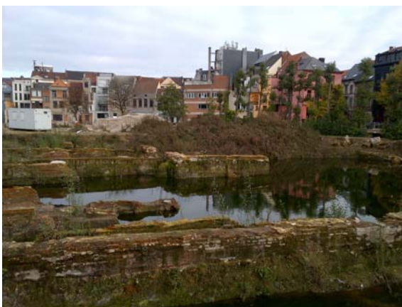
Photo: The site with demolished buildings before the start of the works.
